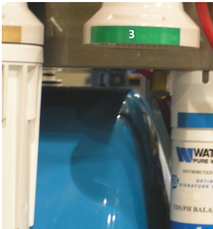
Figure 6-12. RO Membrane Replacement
