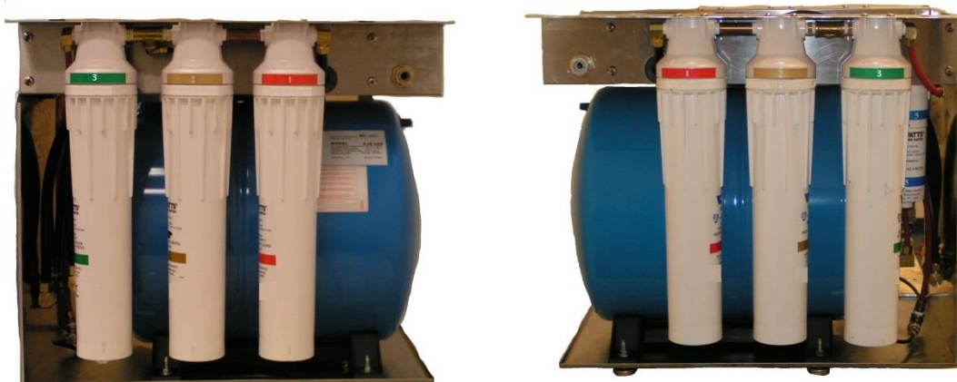
Figure 4-5. Pre-Treatment Filter O-Rings
