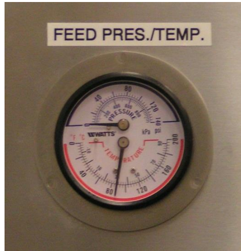
Figure 5-3. Feed Water Temperature
