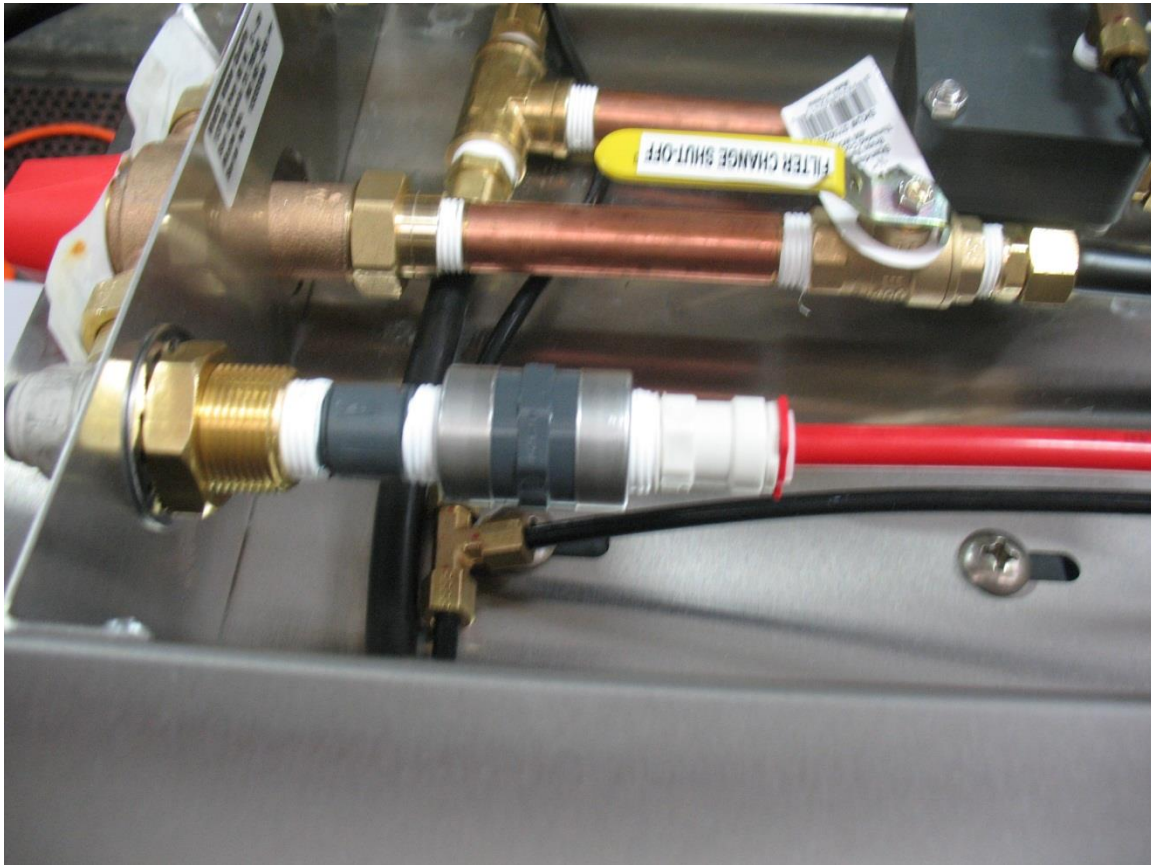
Figure 6-10. Type 3 Flow Control Valve Installed
