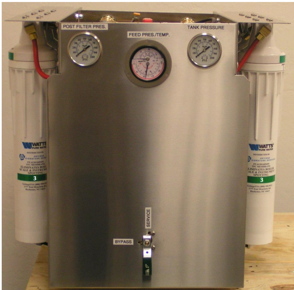
Figure 3-1. HS-333 Water Treatment System
